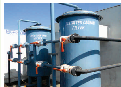
UNIT OF ETP SAND FILTER AND ACTIVATED CARBON FILTER
