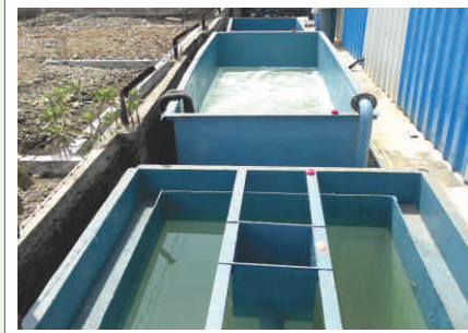
Small Fabricated Low Capacity ETP
