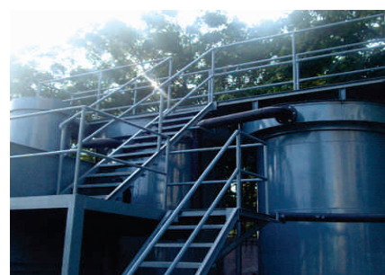
Fabricated Sewage Treatment Plant M/s Hotel Fortune Landmark, Indore
