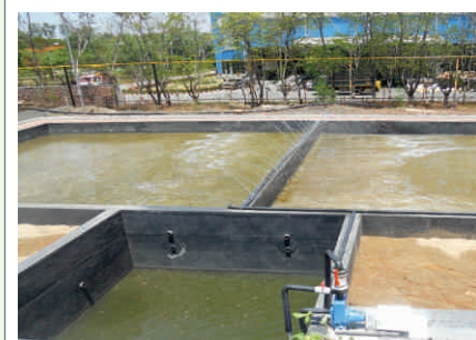
Evaporation Pond for High TDS Water M/s Tata Steel Ltd., Pithampur
